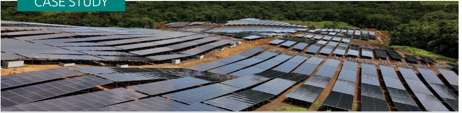
Palau solar plant. Credit: DFAT
